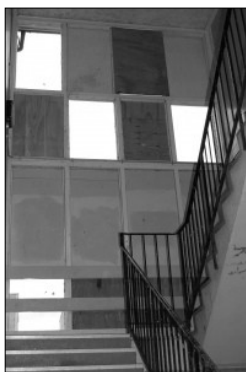
SLE Windows Boarded up
